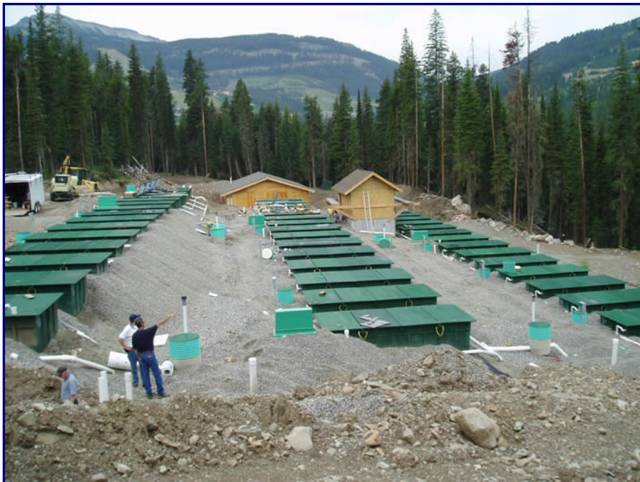
Figure 3 – Large Advantex® Treatment System, Camp Red Cloud, Lake City, CO
